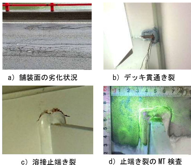
図-1 舗装面劣化状況と溶接止端部の疲労き裂
